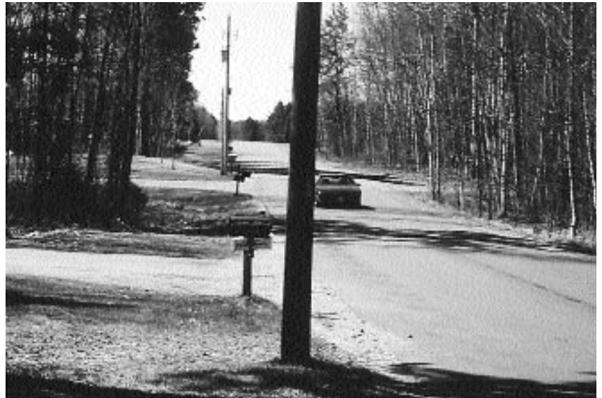
Utility pole located very close to the edge of the shoulder. Relocation to tree line would be desirable.
