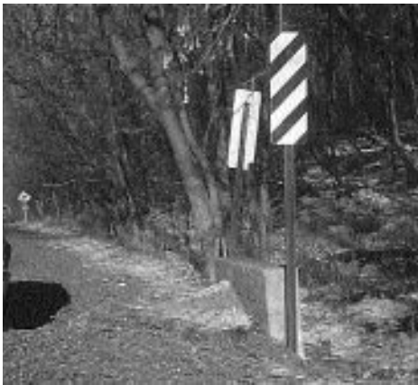
Concrete culvert headwall protruding above the shoulder creates a hazard.
