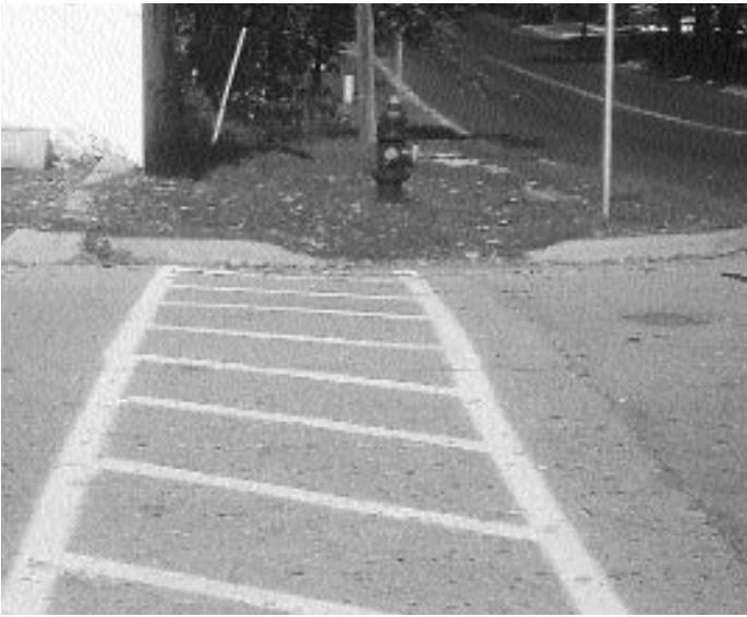
Incorrect crosswalk. Minimum crosswalk width is six feet. Optional diagonal stripes should be at 45 degrees or perpendicular to crosswalk lines.
