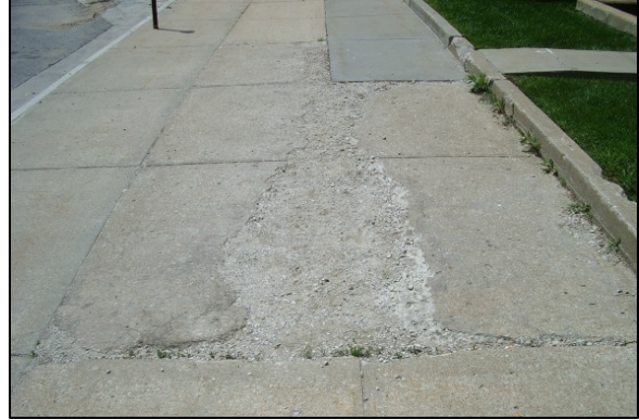
Figure 7: Spalling on a sidewalk
