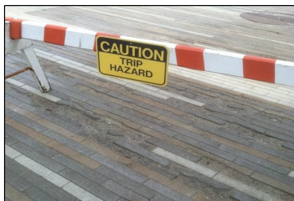
Figure 6: A crumbling surface on this walkway can lead to accessibility issues and tripping hazards.
