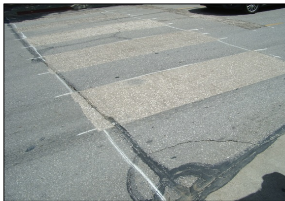
Figure 11: A street is prepared for the installation of new crosswalk in-laid markings.
