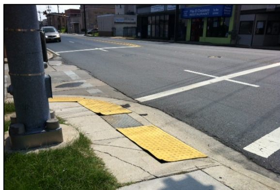
Figure 10: Damaged detectable warning fields.
