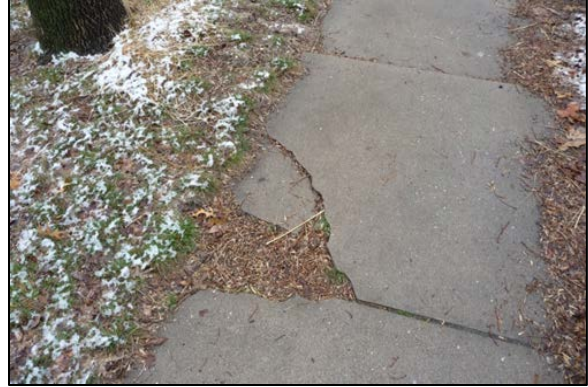
Figure 8: Cracking of sidewalk sections can lead to accessibility issues.
