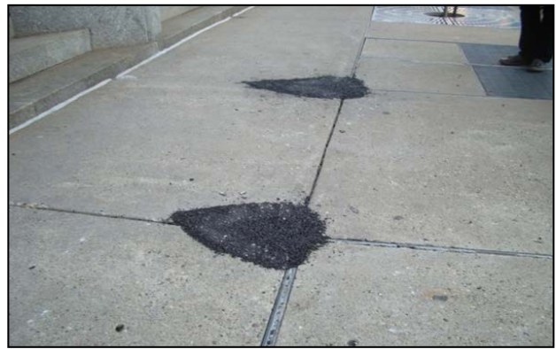
Figure 21: The areas have been temporarily repaired with asphalt patches. Note the patching material overlaid on the concrete extending beyond the hole.
