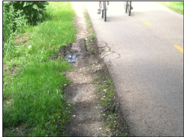
Figure 35: Inadequate shoulders on a path resulting in edge damage.
