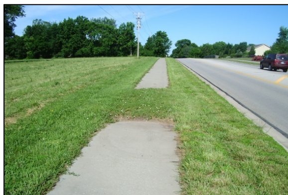
Figure 16: Soil accumulation across a sidewalk has allowed for thick vegetation overgrowth which limits the use of the sidewalk by people with some disabilities.
