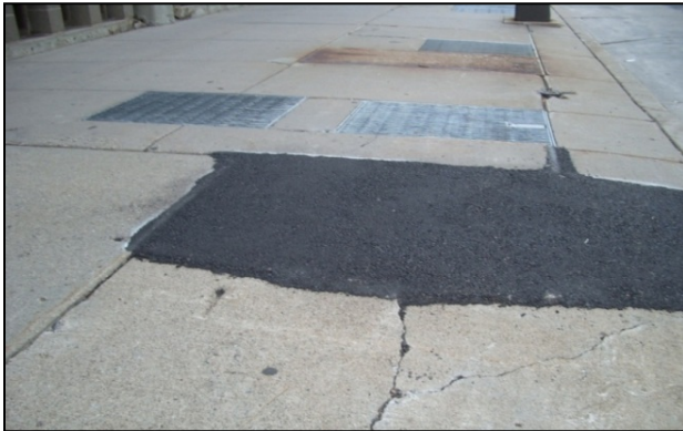
Figure 23: Wedge has been placed to mitigate the hazard caused by a raised sidewalk slab. Note the extensive and appropriate ramping of the wedge.
