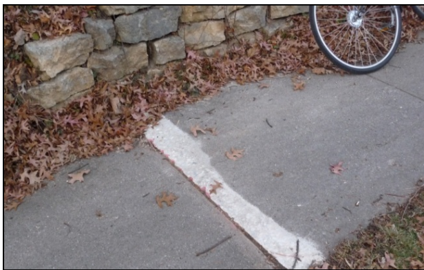
Figure 25: A raised sidewalk block has been ground down to provide a smoother transition.
