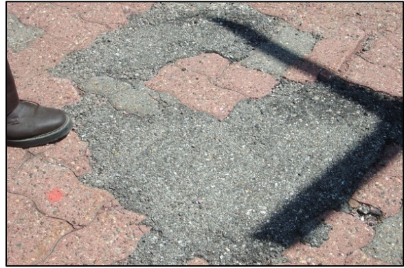
Figure 29: Damaged pavers have been repaired with asphalt to alleviate a hazard.
