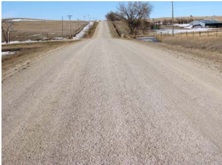
Example of very good surface gravel that has performed very well through the winter in the northern high plains.
