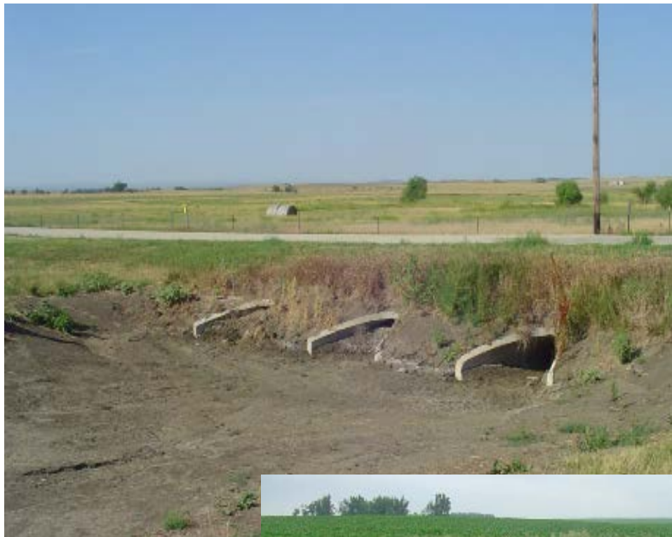
Good work in progress to clean soil from ditch and existing culverts.
