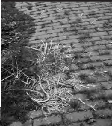
Grass in open joints.
