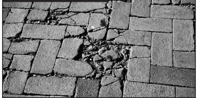
Open joints and broken brick at utility cover.
