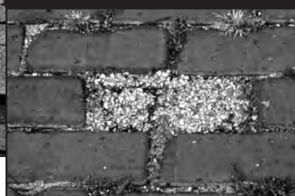
Patch for missing brick.
