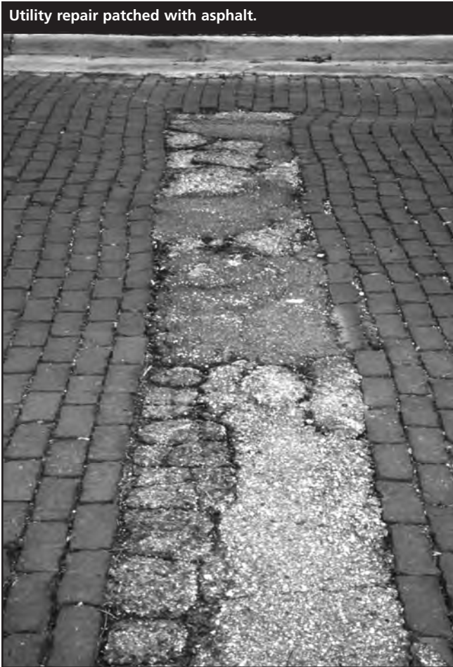
Manhole repairs leaving surface in very poor condition.
