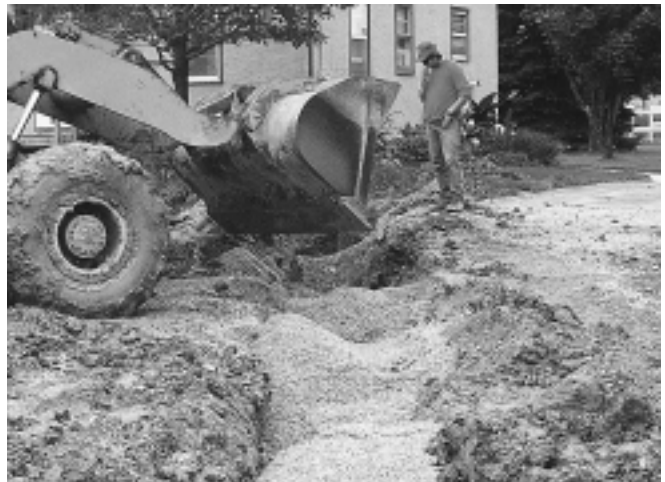
(TOP) Reclaimed glass, crushed to 3/8 inch, unmixed with aggregate is used as backfill over storm sewer. CTH J Brown County.
