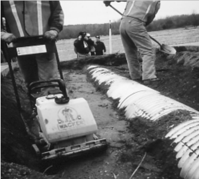
Compacting backfill blend of broken glass and aggregate in culvert trench. Dodge County Highway Department.
